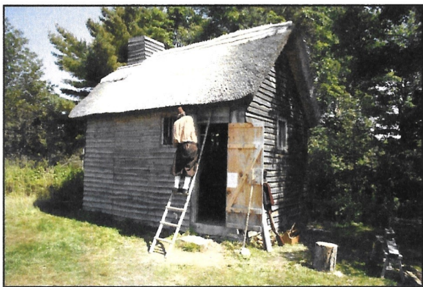
Reproduction of a 17th Century fisherman's home, typical of those found in New England, under construction.
